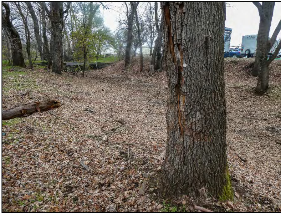
Tree #31 has a long wound in the trunk exhibiting evidence of rot and a severe uneven weight distribution Photo Date 01-20-20.
