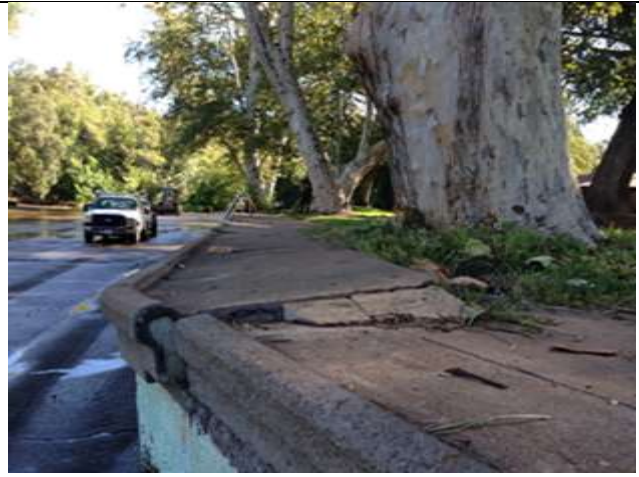
Figure 2. Tree roots have lifted up the pool deck. The asphalt repair has helped but has deteriorated as well.
