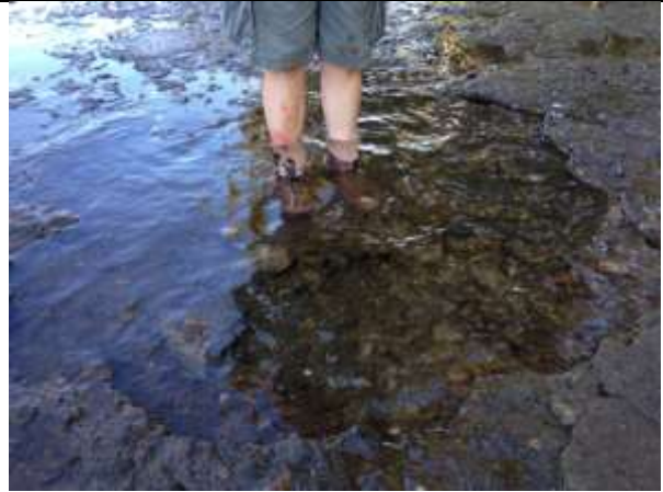
Figure 4. Pot-holes in the base of the pool may expose swimmers to injury, and may erode more, further threatening the integrity of the pool.
