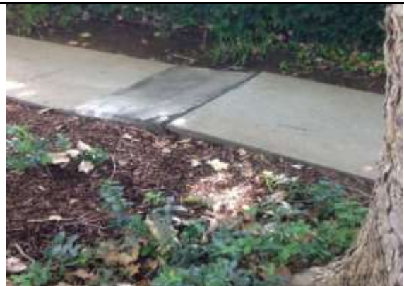
Ramping the raised sidewalk with asphalt is a temporary fix.
