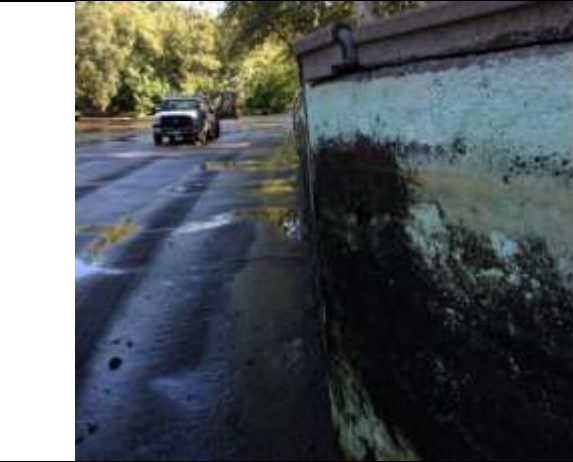
Figure 3. Tree roots have also pushed out the wall which is now leaning 6° into the pool. The repair may slow down the collapse of the wall, allowing enough time for devising a more permanent long-term fix.
