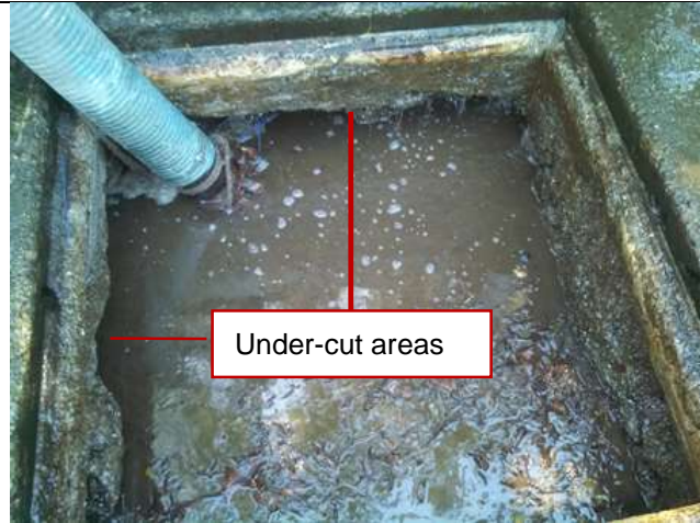
Figure 1. Water has eroded the substrate around the base of the vault. Continuing erosion will threaten the bottom of the pool.
