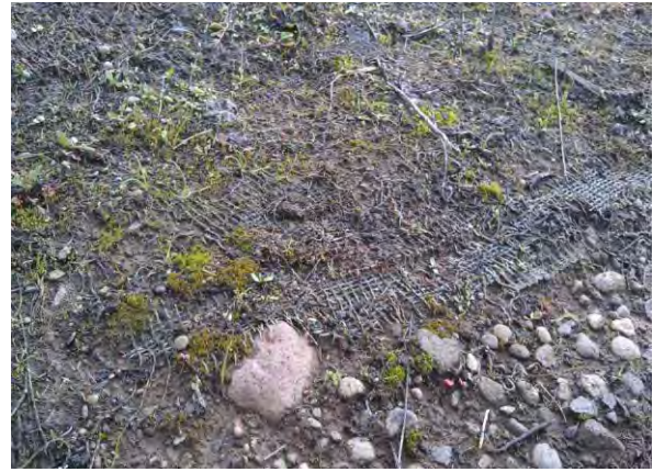
Photo 2: Exposed landscaping fabric along western landfill area.
