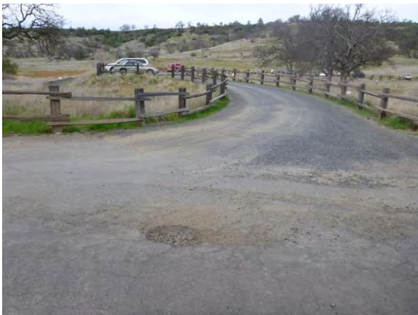
Photo 5: Parking lot entrance (view north) exhibiting potholes.
