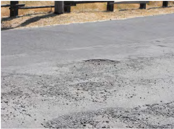
Photo 3: Pothole at the parking lot entrance
