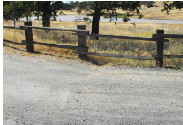
Photo 4: Possibility of erosion due to channelized runoff at the entrance to the parking lot
