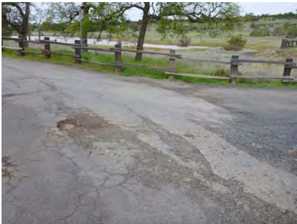
Photo 3: Deteriorating road surface and transition to parking lot apron.
