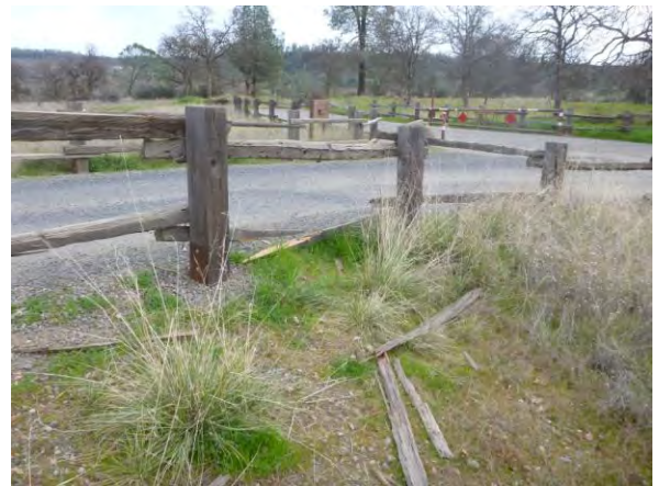
Photo 6: Panel of broken fencing near parking area entrance.
