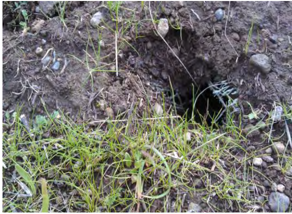
Photo 1: Rodent burrow through landscaping fabric near monitoring sump.
