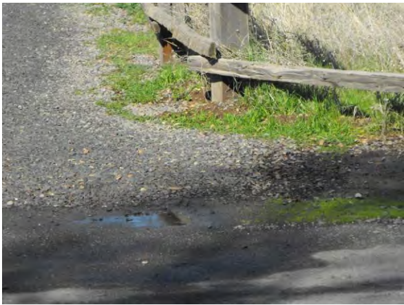
Photo 3: Ponding water in pot hole near parking lot entrance.
