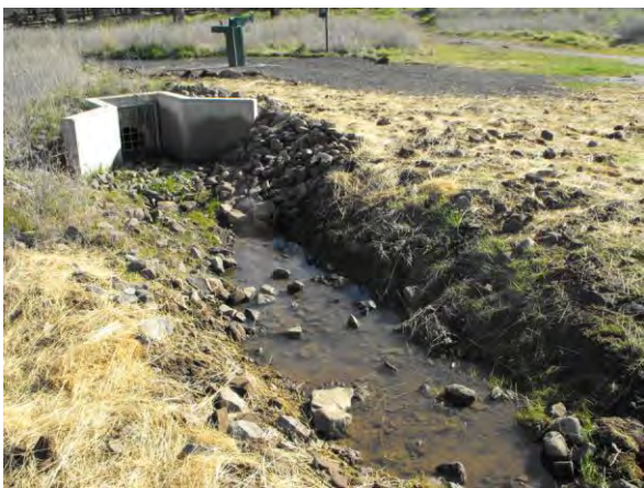
Photo 5: Pipe outlet overview (ponded water, sample not collected)
