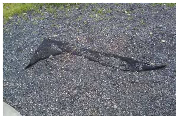
Photo 6: Exposed landscaping cloth along gravel path (outside landfill area).
