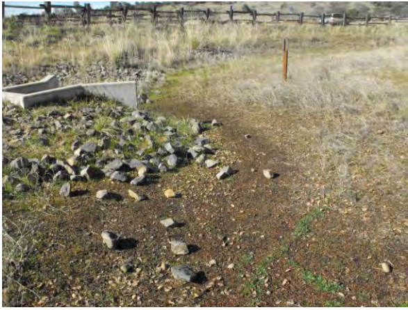
Photo 1: Exposed soil around catch basin insert.
