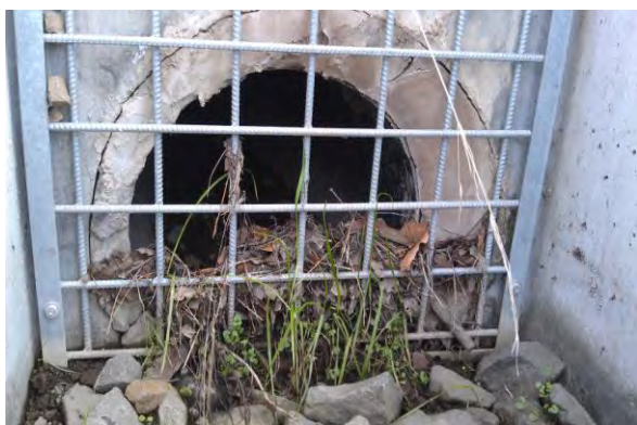
Photo 5: Minor obstructions in drain outlet on south side of parking lot.
