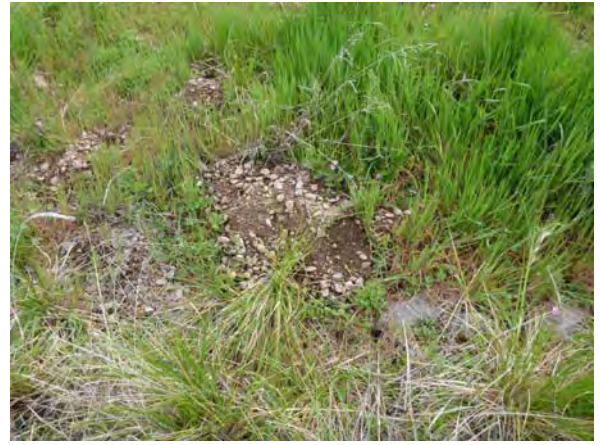
Photo 2: Rodent burrowing by riprap on north-facing slope. Activity was also observed near the northern path and on the west-facing side.
