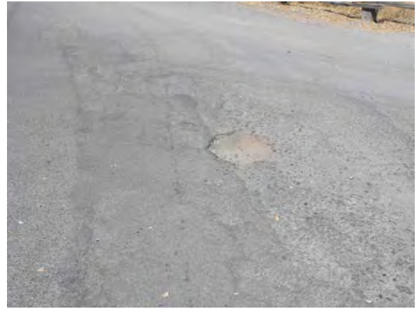
Photo 2: A pothole is present at the entrance to the parking area.
