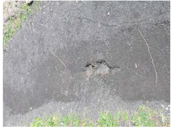
Photo 2: Evidence of erosion along main footpath.
