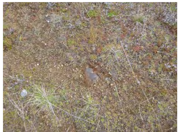
Photo 6: Exposed geotextile cloth on west-facing slope of the cell.
