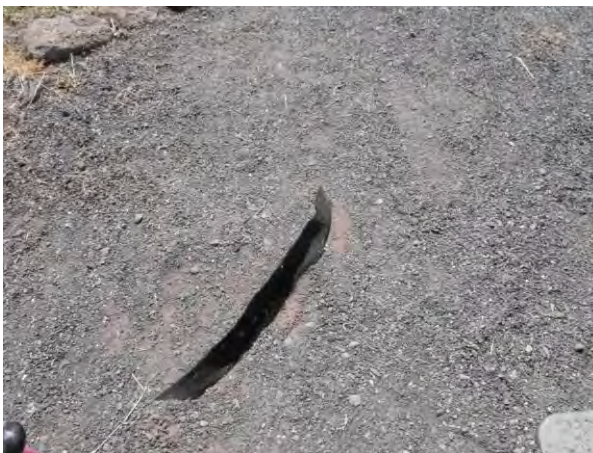
Photo 5: Erosion control cloth is exposed on the trail west of the parking lot
