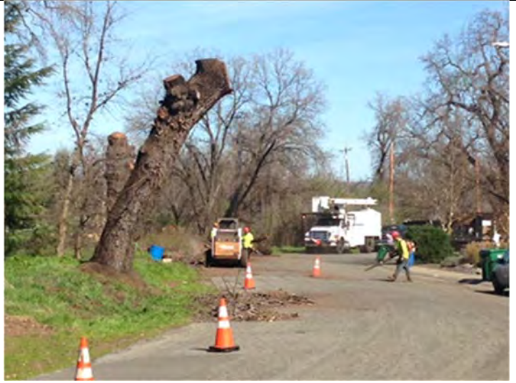
Figure 2 Twin Cities Tree Service the City tree removal contractor removing 3 dead black walnuts at 1281 E Lindo Ave.
