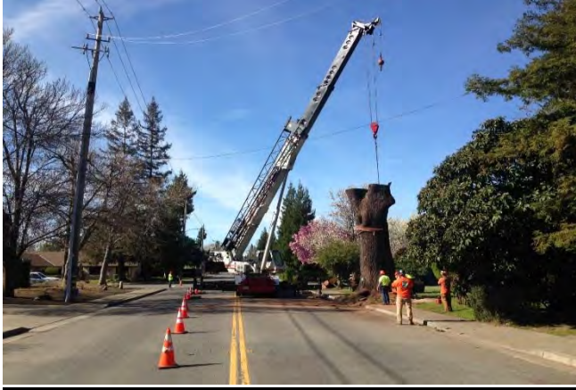
Figure 1. Twin Cities Tree Service removing a dead Black Walnut street tree at W Shasta Ave on 3-8-17.
