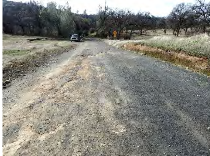
Figure 7. Roads that are flat in cross section, with an outside berm and inside ditch, intercept do not allow the runoff to leave the road. Concentrated road surface and ditch runoff flows down the road with increasing velocity and discharge, creating surface erosion, rills and gullying.
