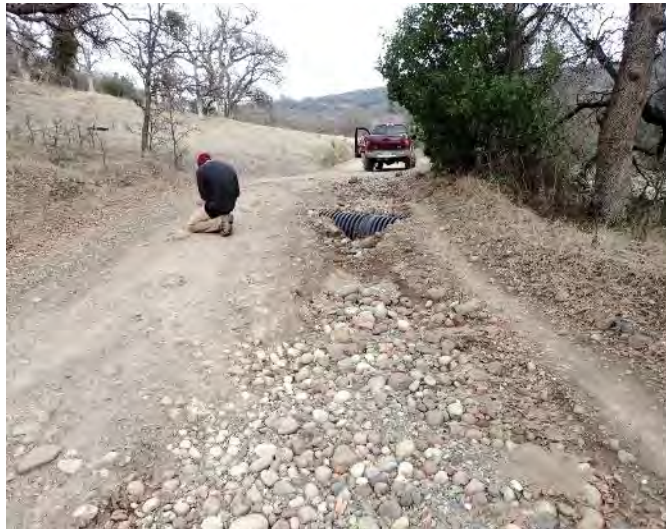
Figure 2. At feature #27 the stream crossing culvert is exposed by erosion cause by an active road surface gully.
