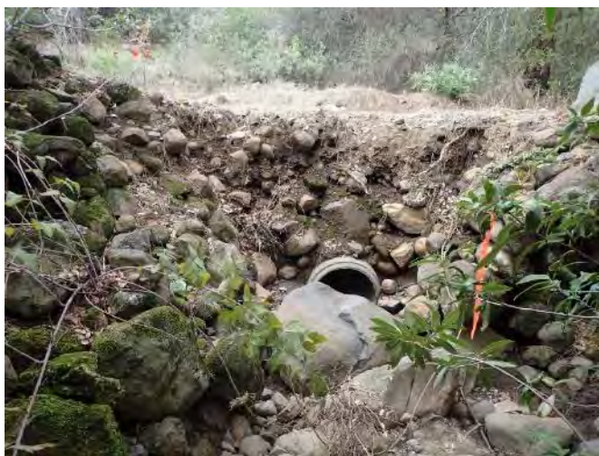
Figure 1. This stream crossing site is plugged by a boulder that dwarfs the concrete culvert inlet. The culvert is undersized for the upslope drainage area and was assigned a high priority for treatment.
