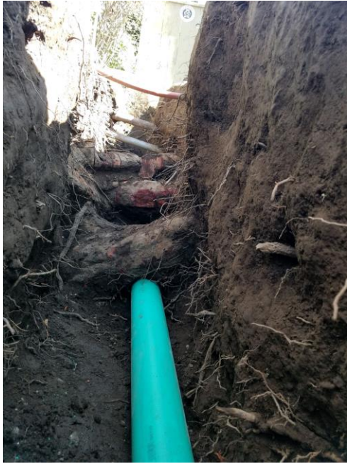
Photo 3: Sewer lateral repair on Wall St. Replacement pipe was placed under tree roots in the trench. Roots were not cut.
