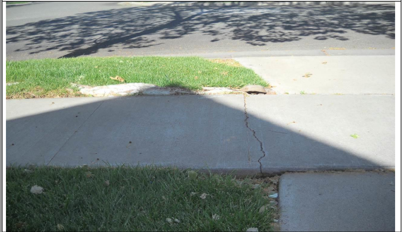
Sidewalk damage from the invasive roots.
