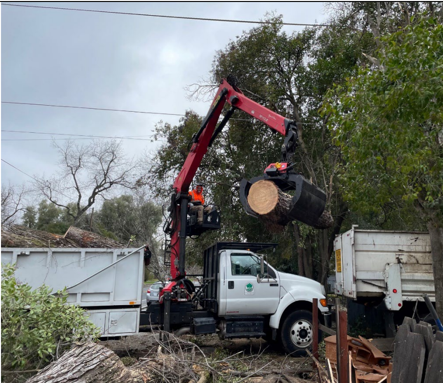
Figure 3- City tree crew storm damage cleanup.
