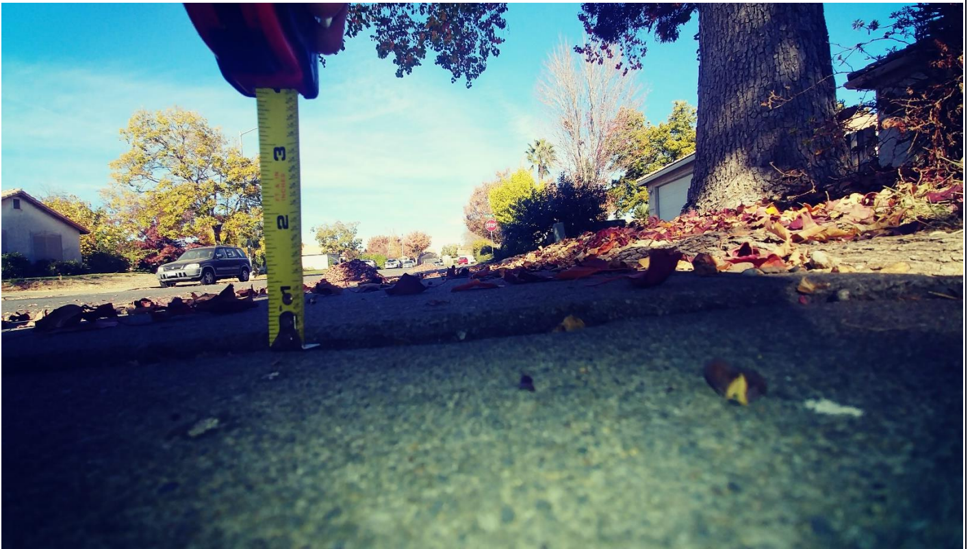
Figure 9. Sidewalk lift is ¼".
