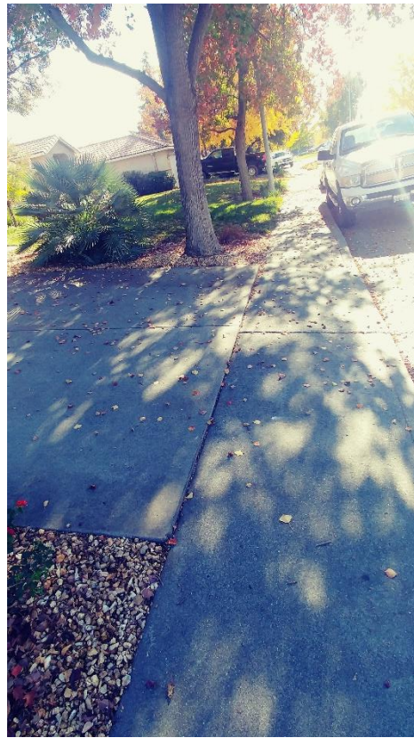
Figure 5. Driveway is partially lifted
