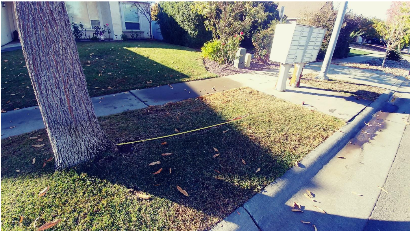
Figure 8 Tree and vicinity to mailbox. Tree is 12' away. Minor slab lift is noted on the adjacent mailbox located in the park strip
