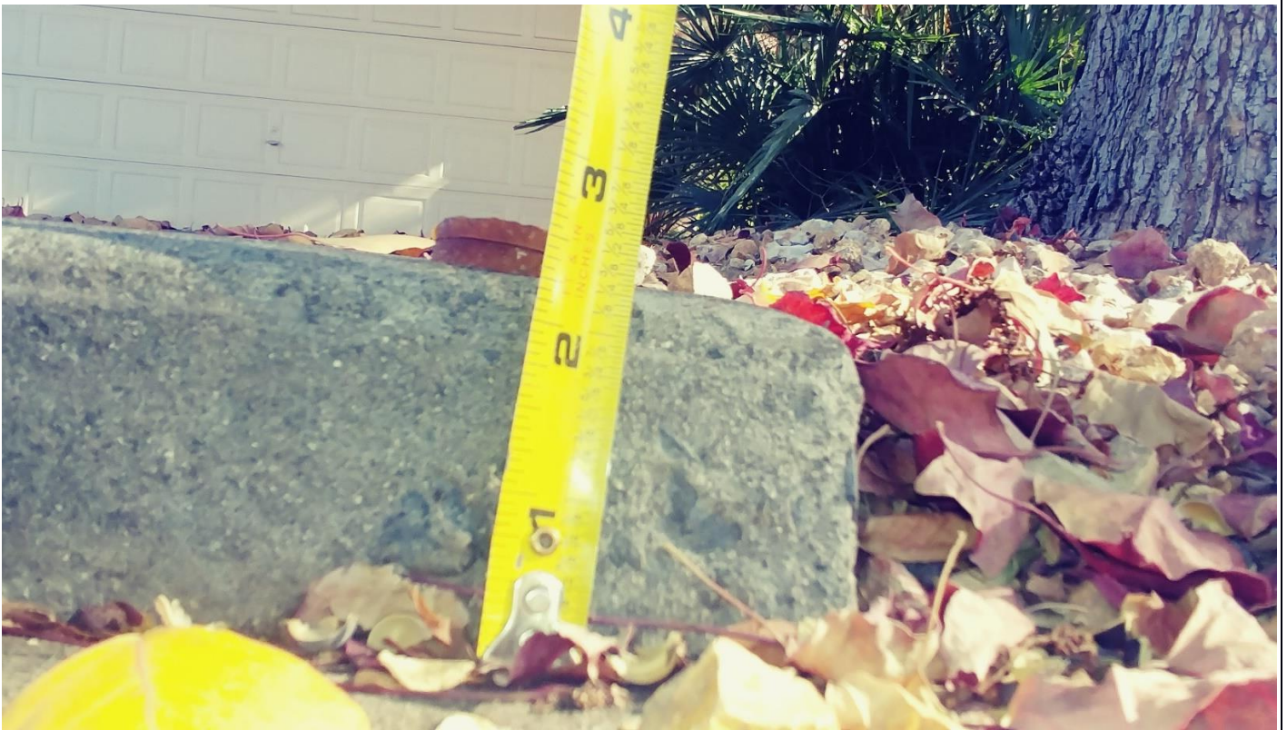
Figure 8. 2 ¼" driveway slab lift
