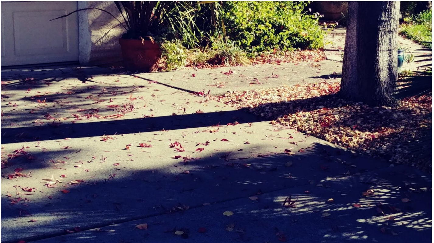
Figure 3. Minor slab lift observed near ash tree located on property.
