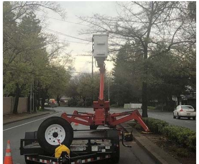
Figure 2. M&S Wesley spider lift used in removing dead trees in the central median on 20 th st
