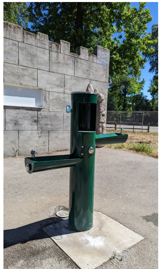
Figure 8 Water-bottle fill drinking fountains
