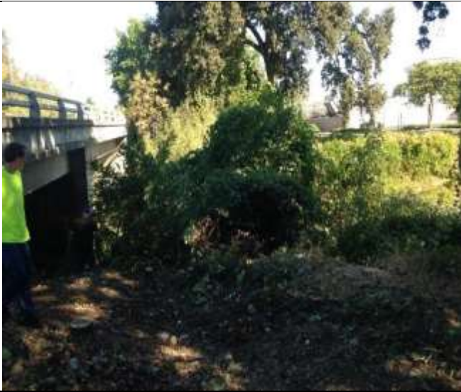
Figure 9. Areas overgrown with non-native invasive vegetation on the Lindo Channel were cleared by the Sherriff's ACS Crew and
