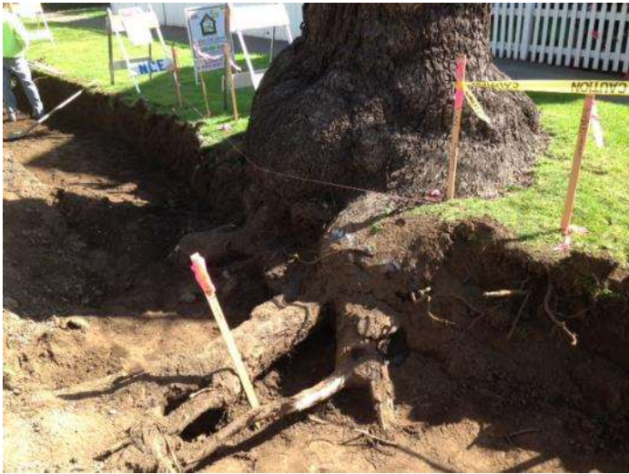
Figure 27. Black Walnut tree was saved by performing selective root pruning and rerouting curb and gutter during construction phase. 1462 Arcadian Ave
