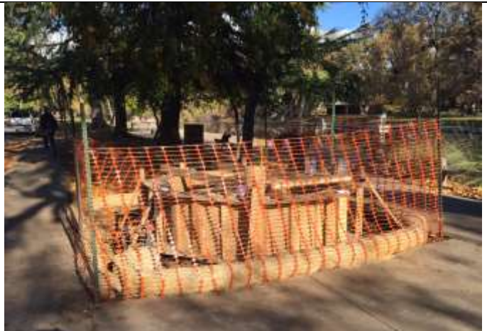
Figure 2. Construction begins on the "Decide and Ride" art installation at the One Mile Recreation Area.
