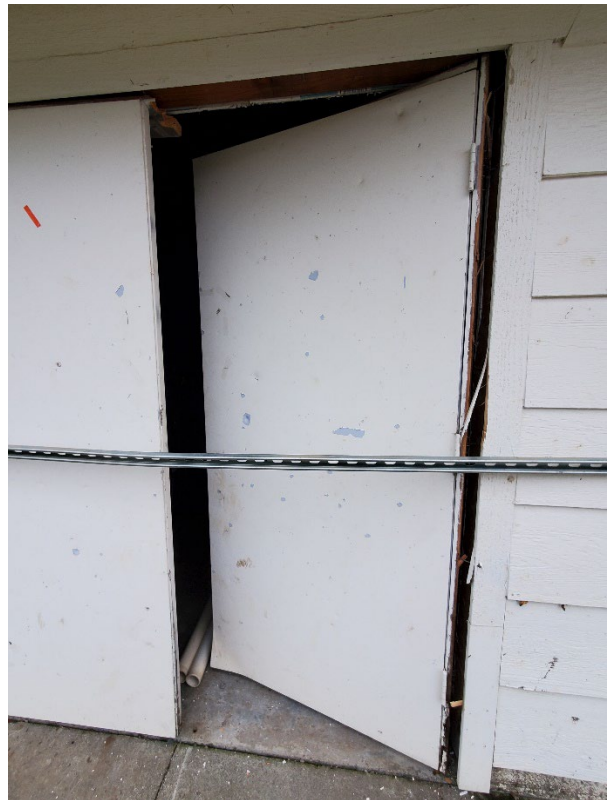
Figure 4: Numerous break ins into Clubhouse
