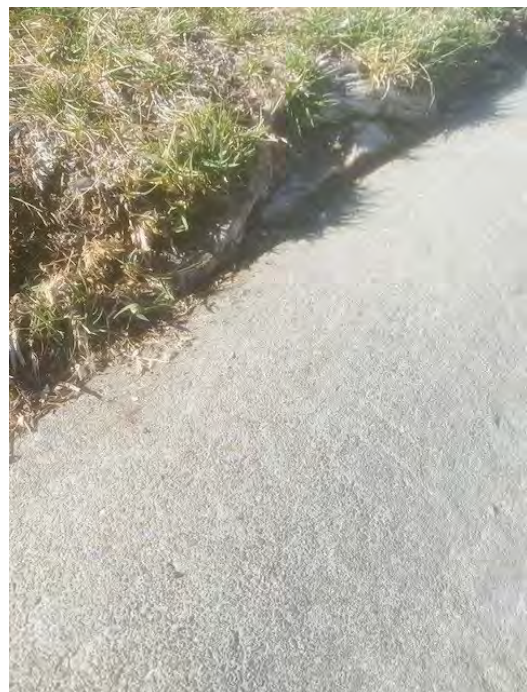
Figure 7. Roots adjacent to sidewalk
