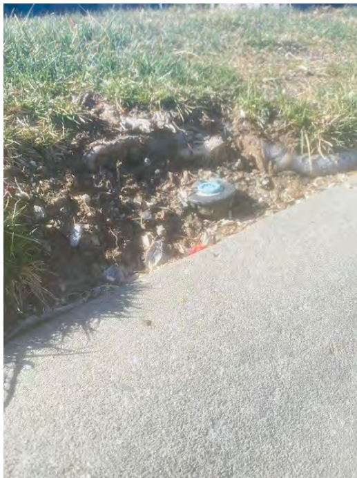
Figure 6. Sprinklers impacted by roots.
