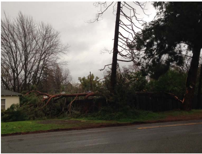
Figure 5. 2117 Zuni Ave a large pine tree limb split and landed on a house 1-18-17.
