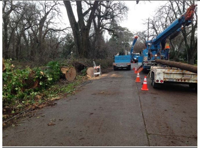
Figure 4. 1351 Woodland Ave PWD cleared the street for PG&E to install a new pole and repair the down wires. Street Trees/Parks then did the final cleanup of wood and debris.
