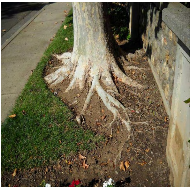
This sycamore in the F:3 position displays invasive roots that are starting to raise the sidewalk that has been replaced once before.
