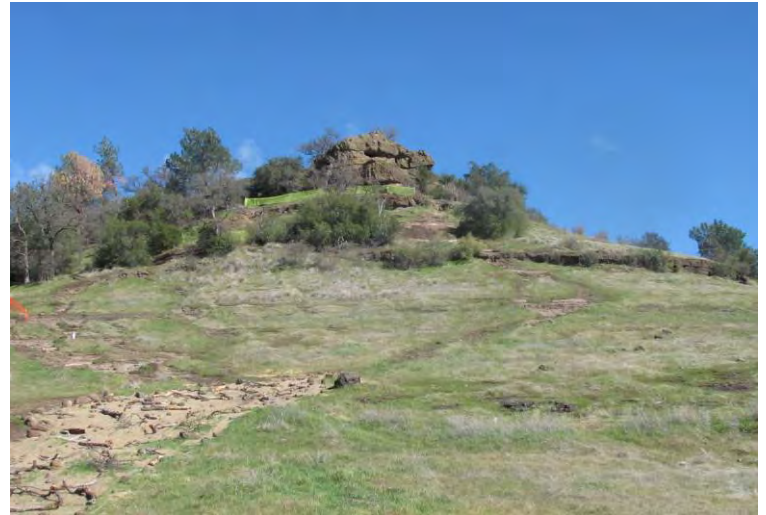
Bidwell Park's "Monkey Face" In the foreground, the installation of jute matting and native grasses to repair scarred eroded trail.
