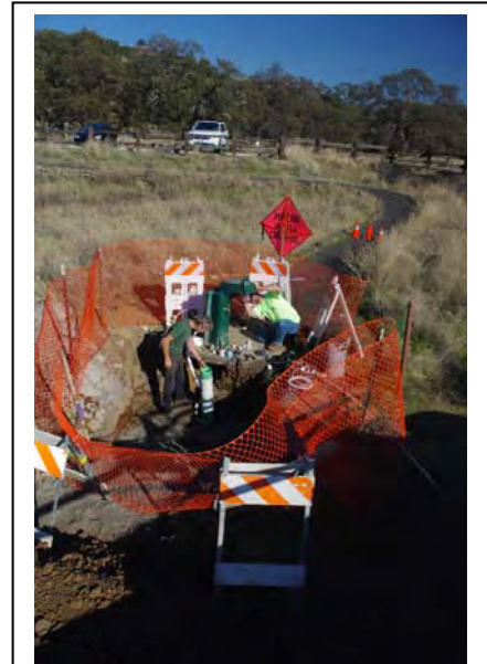
Crew installs French drain to accommodate donated all-weather water fountain at parking lot E.
