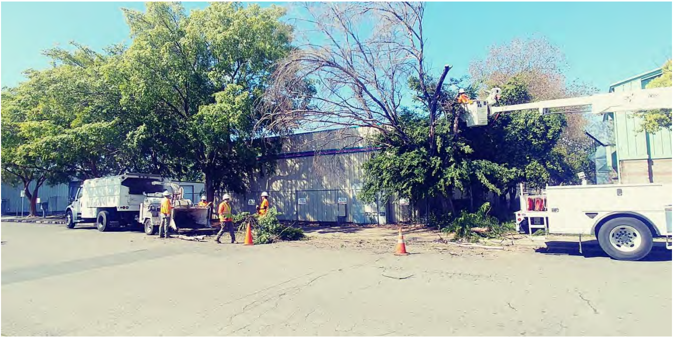
Photo 3. Public Works working on Martin Luther King removing dead pistache tree. March 2020
