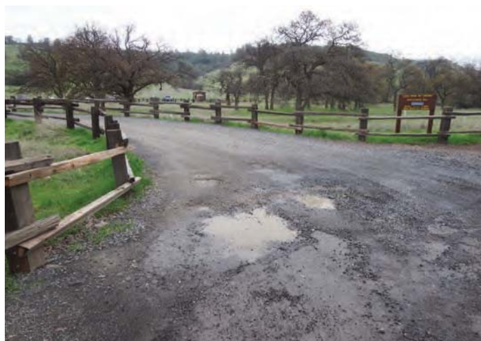
Photo 2: Potholes observed in parking lot area entrance (view northeast)
