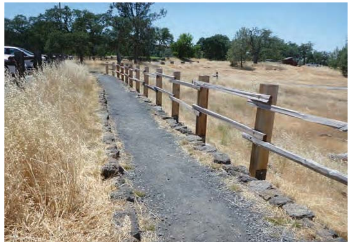
Photo 6: Rilling along footpath adjacent to north central extent of cell has been corrected (view southwest)
