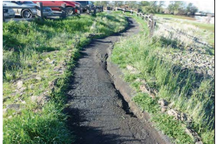
Photo 6: Evidence of rilling along footpath adjacent to north central extent of cell (view southwest)
