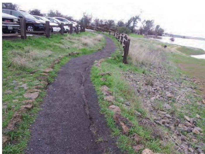
Photo 6: Rilling along footpath adjacent to north central extent of cell
