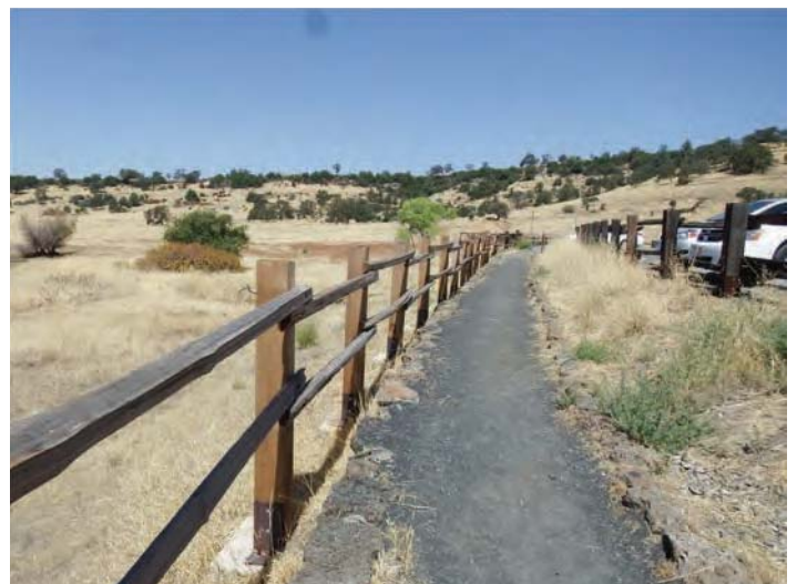
Photo 6: Rilling along footpath adjacent to north central extent of cell has been corrected
