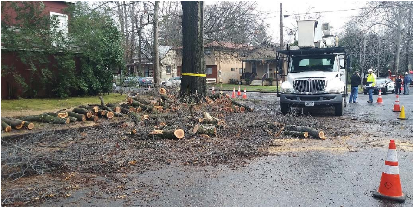
Figure 10. Jan 9, 2019. 742 W 6 th St. Report of PG&E contractor conducting an unauthorized removal. UFM issued stop notice. Chico Police and Code enforcement on scene
