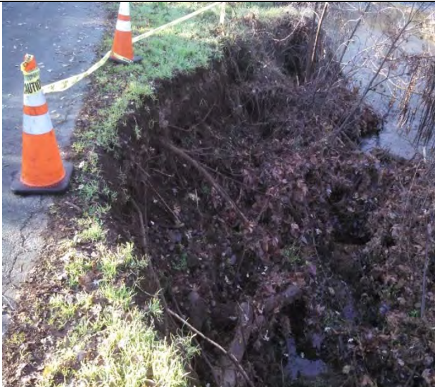
STORM DAMAGE TO SOUTH PARK ROAD
