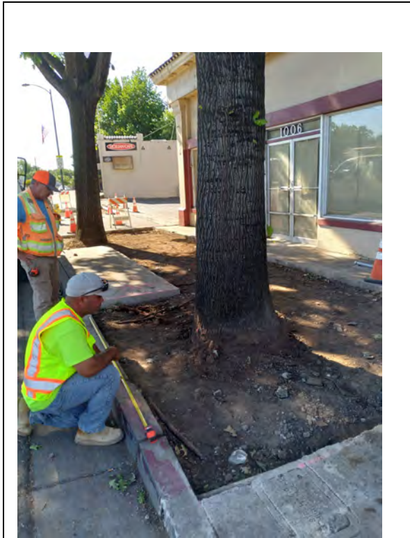
Photo 1 Staff and contractor personnel from Knife River. Onsite discussion to save large tree on Oroville St during sidewalk repair work
