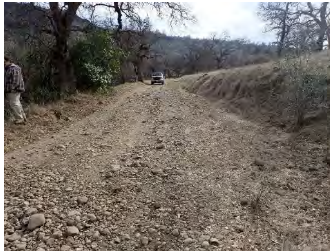
Figure 8. On Upper Park Road a berm has formed after years of grading and road surface erosion. The berm captures and concentrates road runoff, preventing it from being dispersed onto the hillside, and accelerates road surface and ditch erosion rates.
