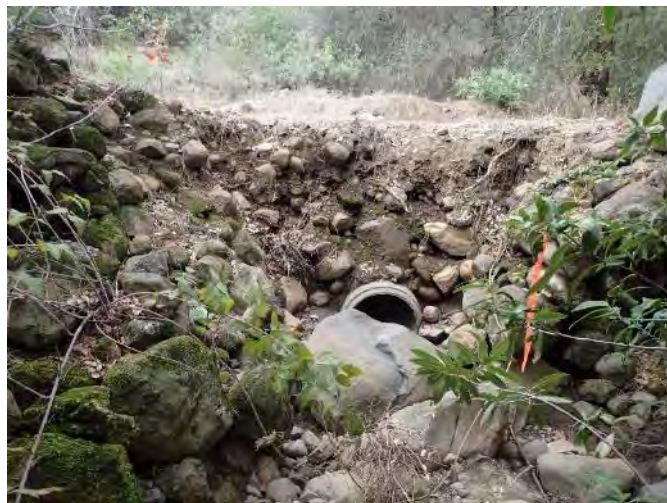
Figure 1. This stream crossing site is plugged by a boulder that dwarfs the concrete culvert inlet. The culvert is undersized for the upslope drainage area and was assigned a high priority for treatment.
