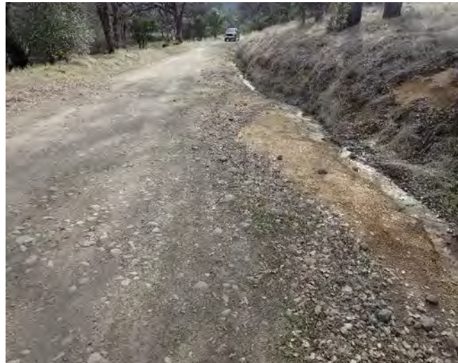
Figure 6. Road surfaces, berms and ditches capture and transport hillslope runoff and direct rainfall during storms. Road surface and ditch runoff often flow down the road grade and directly into stream crossing culvert inlets.
