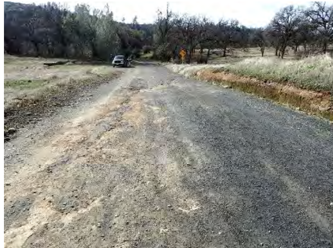
Figure 7. Roads that are flat in cross section, with an outside berm and inside ditch, intercept do not allow the runoff to leave the road. Concentrated road surface and ditch runoff flows down the road with increasing velocity and discharge, creating surface erosion, rills and gullying.
