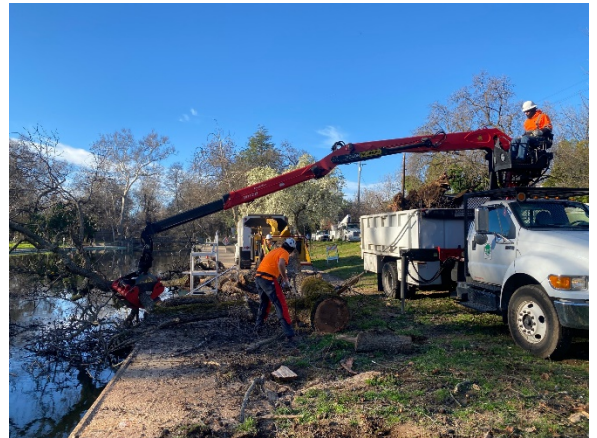
Figure 2: Tree Crew cleaning up fallen oak at One mile
