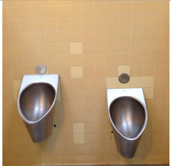
New waterless urinals have been installed at the Five Mile Recreation Area.
