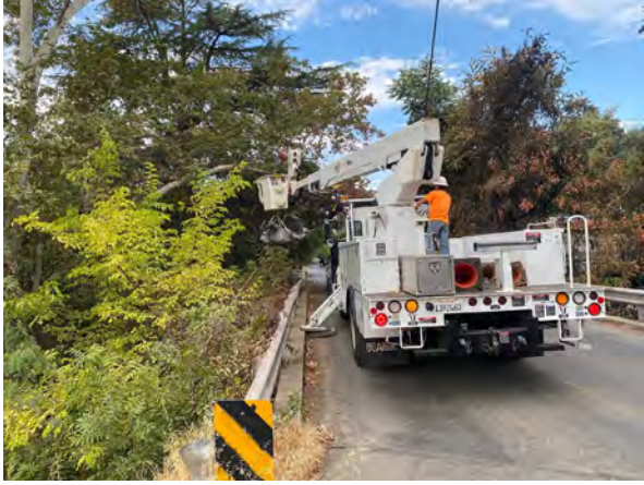
Photo 2. Tree Crew working on Bruce St. Safety prune of tree over the bridge.
