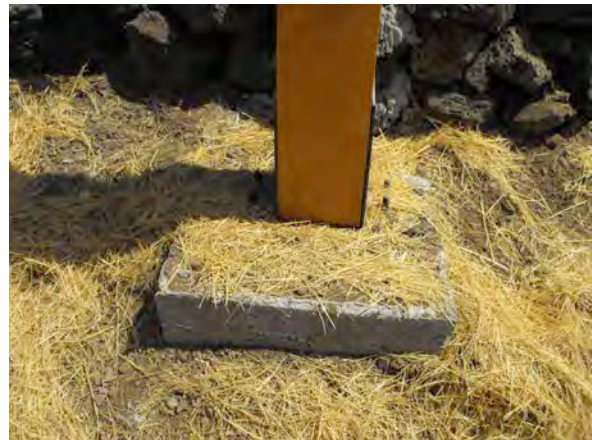
Photo 4: The footing of the fence does not appear to have disrupted the containment cell.
