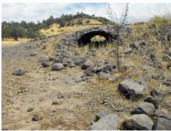
Photo 7: The northern culvert appears to be functioning well, not abnormal erosion was observed around the culvert.
