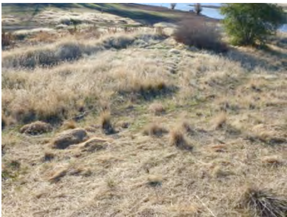
Photo 3: Straw has been applied on the slope of the containment cell and appears to have significantly reduced erosion.
