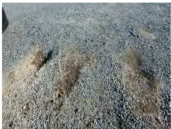
Photo 6: Minor potholes in mid-eastern portion of parking lot
