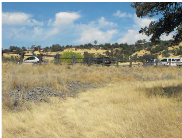
Photo 9: The eastern edge of the containment cell appears to be in good condition.
