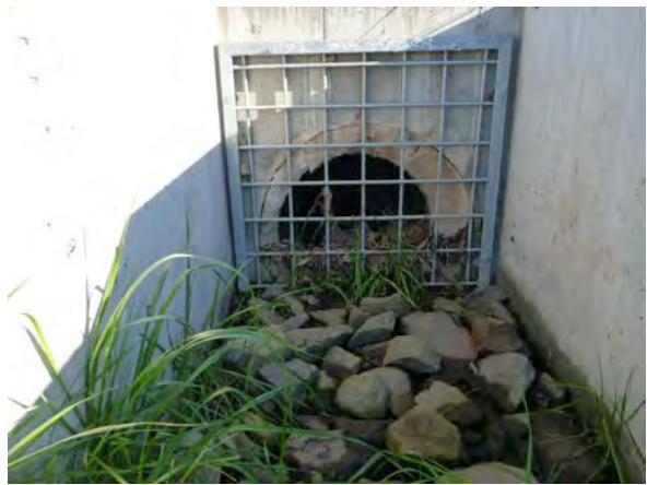
Photo 4: Minor debris in pipe outlet
