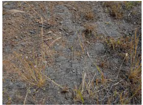
Photo 4: Landscaping fabric showing through on northwestern slope.
