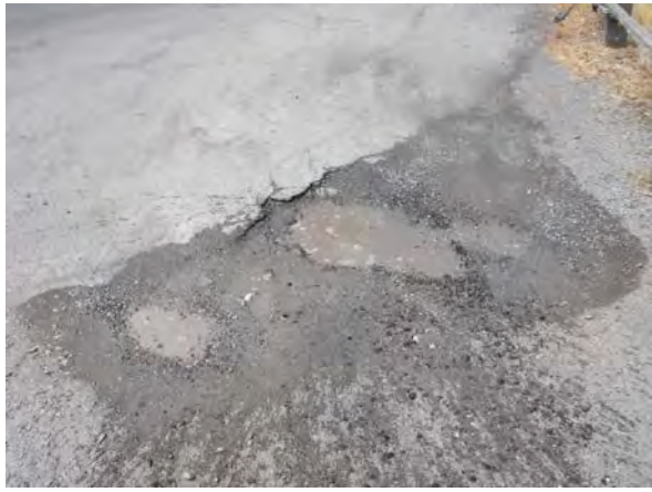
Photo 1: Ponded water in pothole entering the Horseshoe Lake parking lot.
