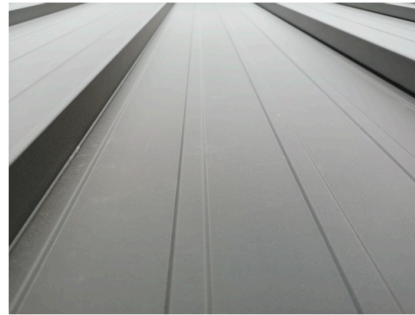
STANDING SEAM METAL ROOF METAL SALES - OLD TOWN GRAY (AT COMMUNITY BLDG.)
