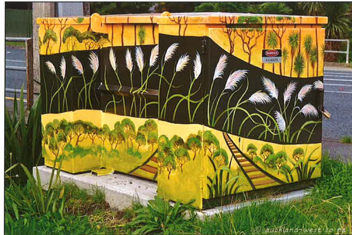
ABOVE-GROUND TRANSFORMER BOX
