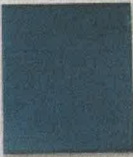
Blue Paint Trash enclosure doors, metal cap flashing, 1x10 stucco trim
