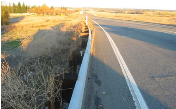
Photo 3. Downstream End of South Fork Dead Horse Slough Along SR 32, Looking West
