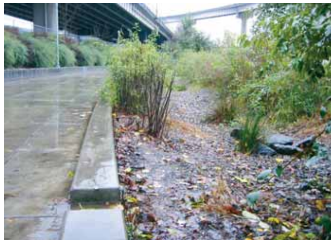
An example of perforated curbs which allow water to infiltrate in a swale.
