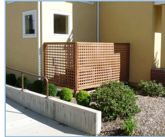
DG 3.1.35- Screened mechanical equipment
