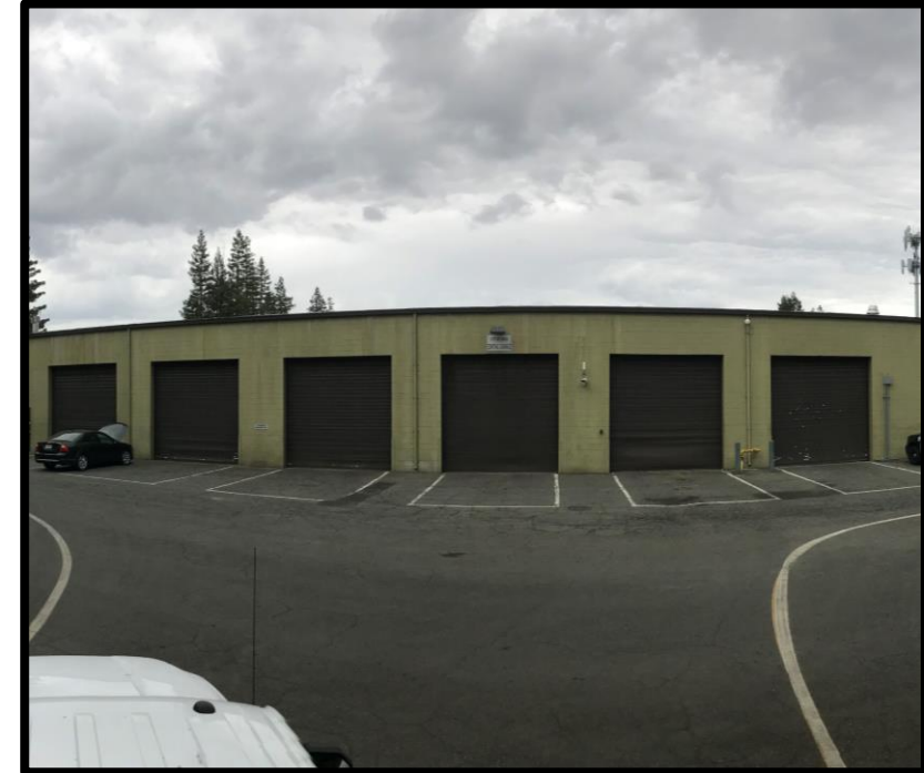
Building 200 Roll-Up Doors
