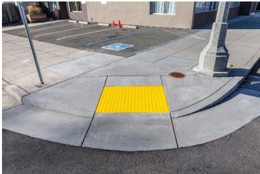
Source: Van Midde Concrete
