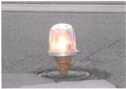
Elevated Runway Edge Light Fixture
