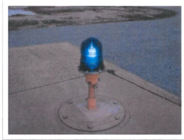
Taxiway Edge Light (elevated)
