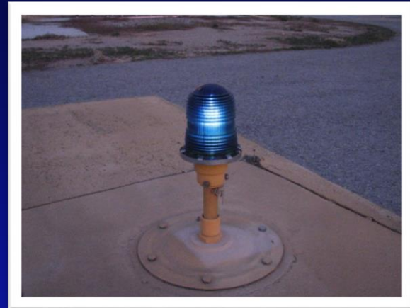
Elevated Taxiway Edge Light
