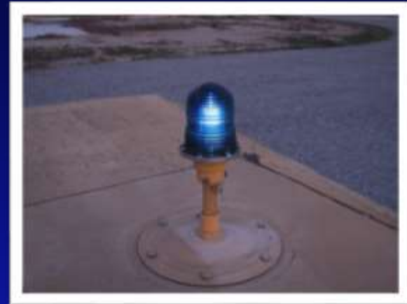
Elevated Taxiway Edge Light
