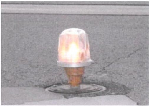
Elevated Runway Edge Light Fixture
