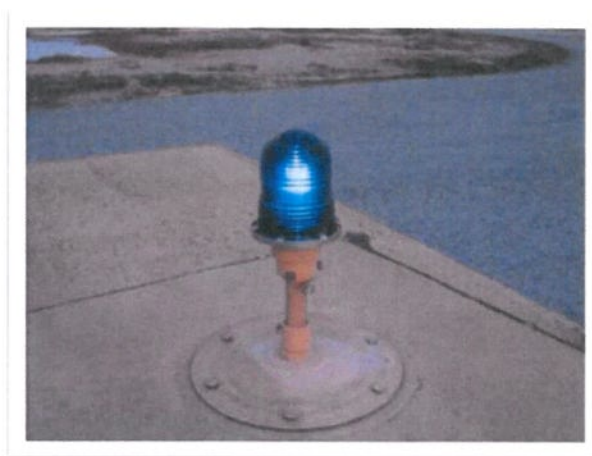
Elevated Taxiway Edge Light
