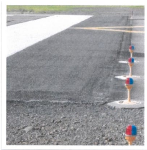
Runway Threshold Lighting
