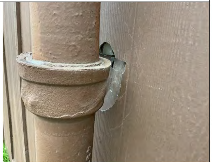
Pipe Damaged by Vehicle
